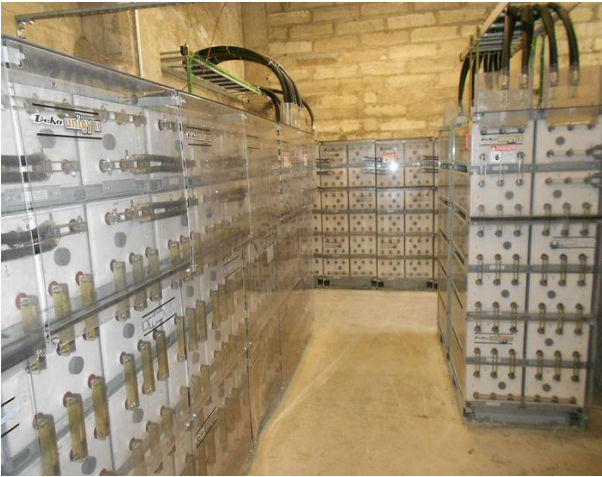
Figure 8. Battery Energy Storage
