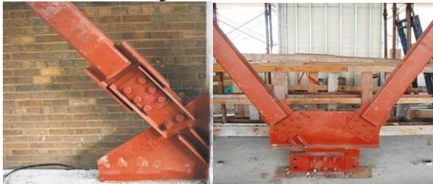
Figure 2. Friction damper in single diagonal bracing Figure 3. Friction damper in chevron bracing (inverted)
