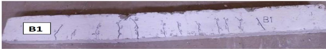
Figure 8.1 Cracking pattern of Beam B1
