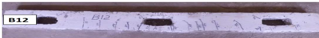
Figure 8.12 Cracking pattern of Beam B12
