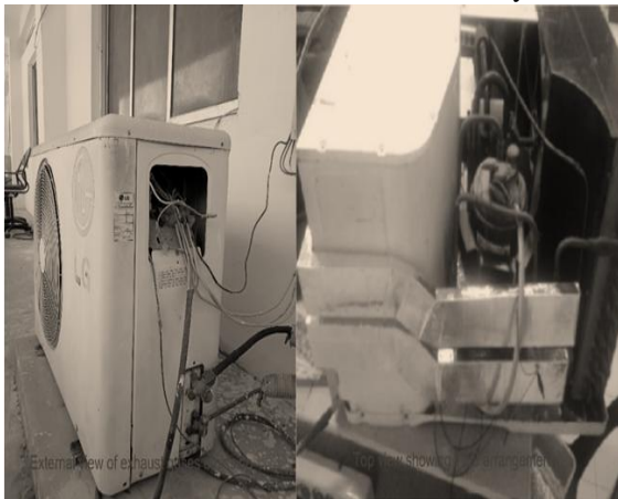
Fig. 5. TEG Arrangement Fitted To The Exhaust Of Air Conditioner
