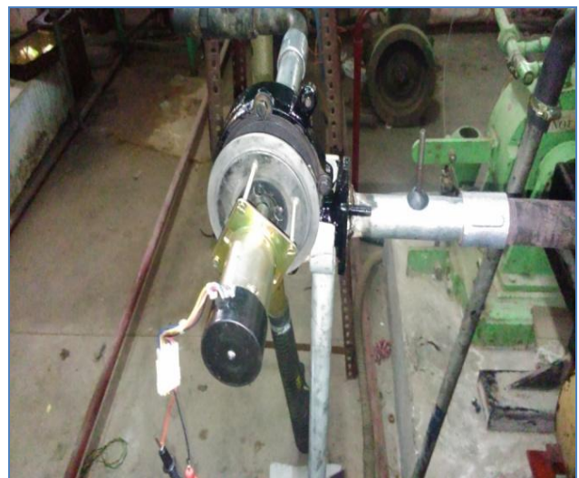
Figure 4. Shows generator coupled
