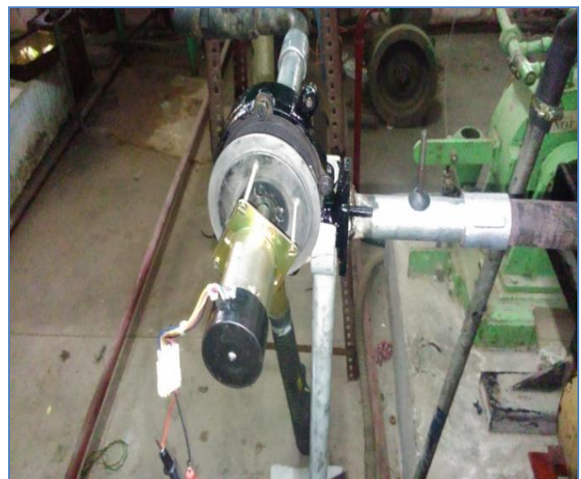
Figure 4. Shows generator coupled
