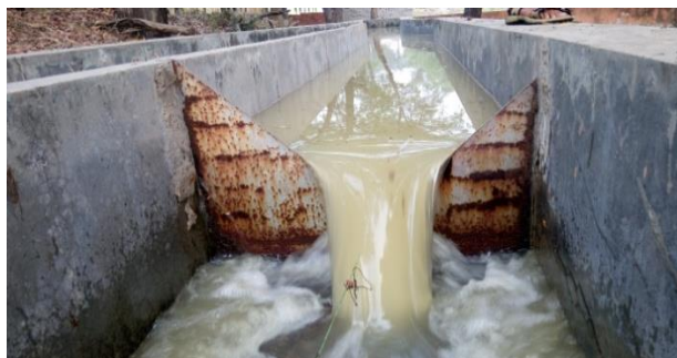
Figure 4: Discharge in V notch
