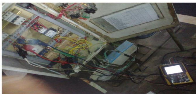
Fig.1. Data Analysis using Power Analyzer
