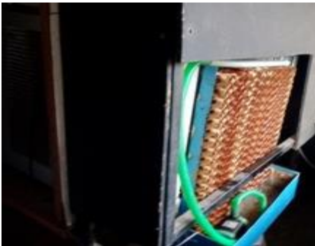
Fig.1 Evaporative cooler attached back side on condenser of Window Air Conditioning Trainer.
