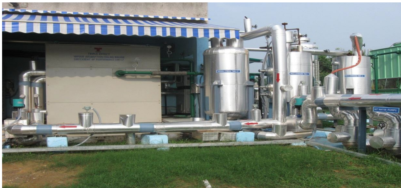
Figure 1. Triple effect vapour absorption cooling system at National Institute of Solar Energy, Gurgaon. The month-wise experimental observations for the triple-effect vapour absorption have been shown in Table 1.
