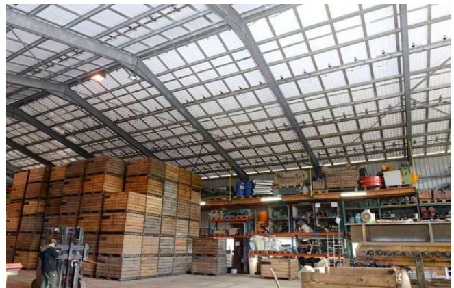
Fig. 6. The transparent photovoltaic panels replaced the cancerogenic Eternit of the farmer warehouse adding brightness to the interior space (from: Mise au Point, 2018)
