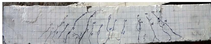
Fig.6 Crack formation in B-3
