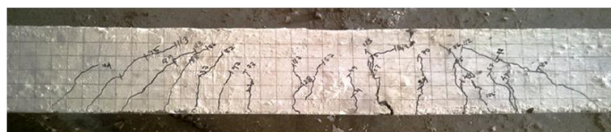
Fig.6 Crack formation in B-4
