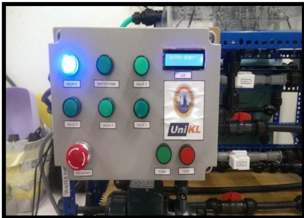
Fig. 9 Indication of the system in ready mode
