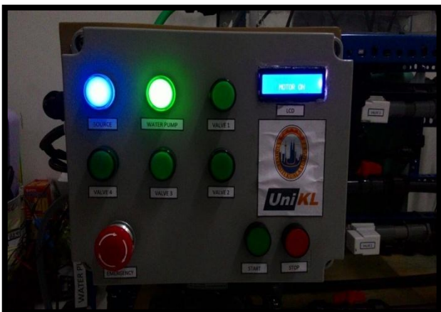
Fig. 10 Pump is on
