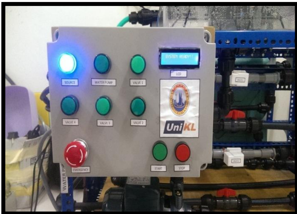
Fig. 9 Indication of the system in ready mode
