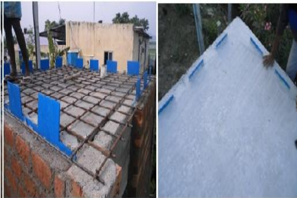
Fig: 2.5 (a) Slab work with fluted sheets projection (b) completion of roof.
