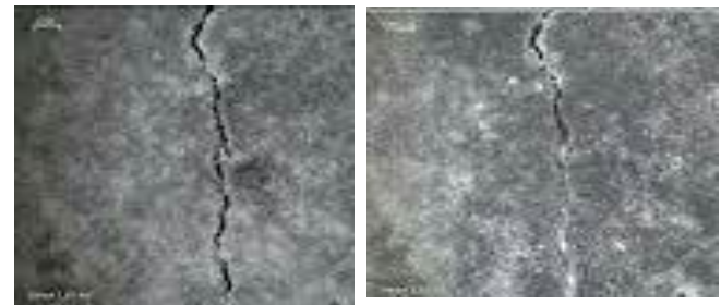
The crack made in the Concrete Cube made up of Bacillus Sphaericus
