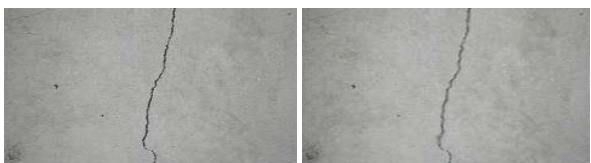
The crack made in the Concrete Cube made up of Bacillus Subtilis
