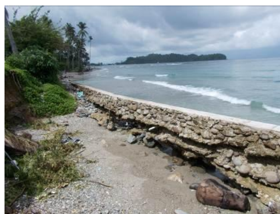
Fig. 1 Ground scour behind the revetment building due to overtopping waves
