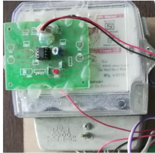
Fig3. Opto coupler connected to energy meter
