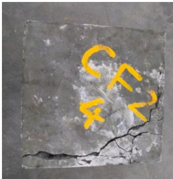
Figure 11 crack observed on three sides supported slab specimen with 0.3% of steel fibre
