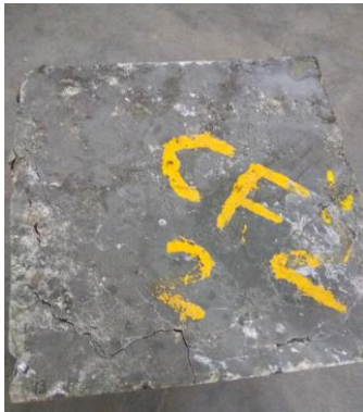
Figure 10 crack observed on four sides supported slab specimen with 0.3% of steel fibre
