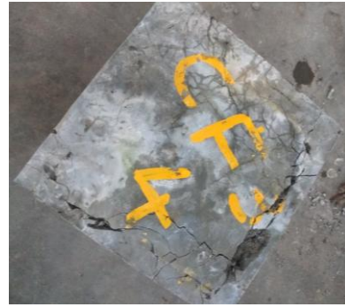
Figure 13 crack observed on four sides supported slab specimen with 0.4% of steel fibre
