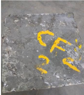
Figure 10 crack observed on four sides supported slab specimen with 0.3% of steel fibre
