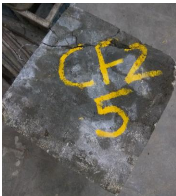
Figure 12 crack observed on two sides supported slab specimen with 0.3% of steel fibre
