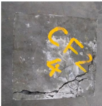
Figure 11 crack observed on three sides supported slab specimen with 0.3% of steel fibre
