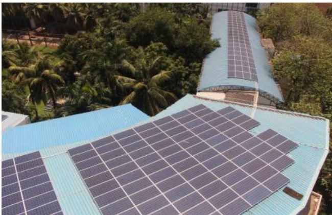
Fig.10: KLEF PV Installations.
