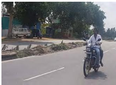
Fig. 13: Damaged median at ch.202.300 Km
