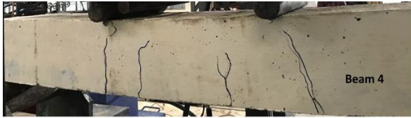
Fig.4e Crack patterns in specimen 4
