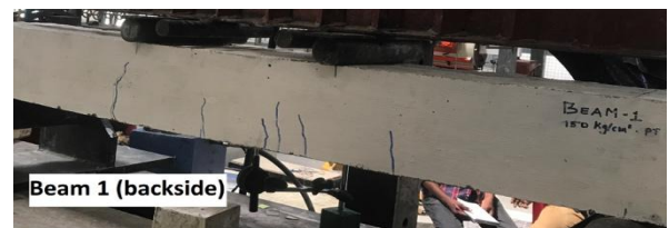
Fig.4b Crack patterns in specimen 1 (backside)
