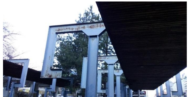
Fig. 1. Structure with corroded steel elements
