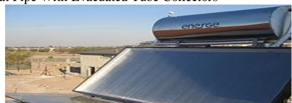
Thermosiphon solar water heater
