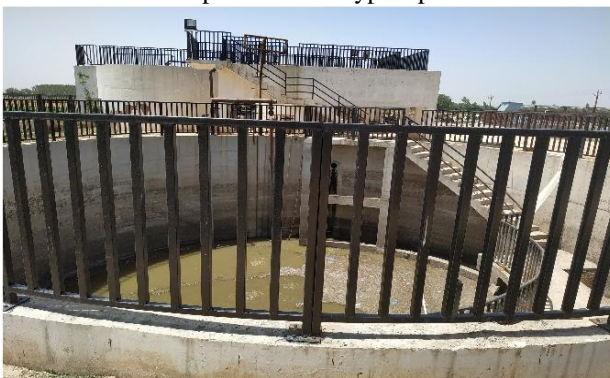
Figure 3. Lehra Sewage Treatment Plant.
