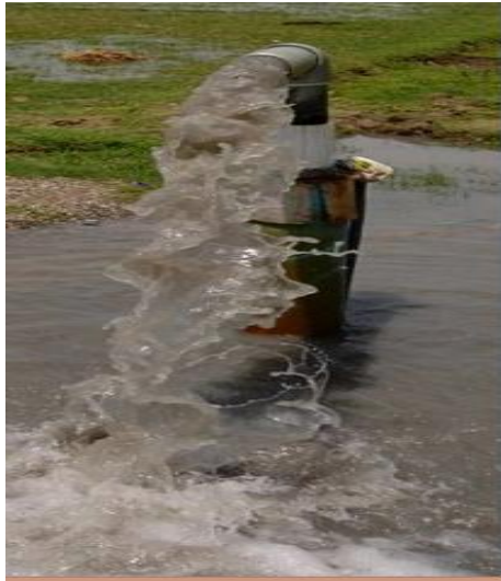
Fig. 4. Installed Water Pump
