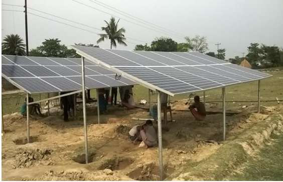
Fig. 3. Installed Solar Panels
