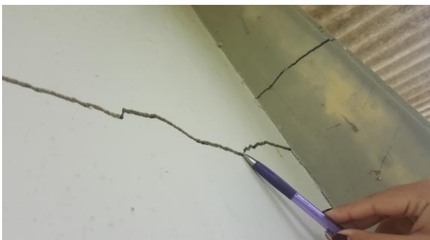
Fig. 11: Foundation Problems (Source: Author's Collection, 2019)
