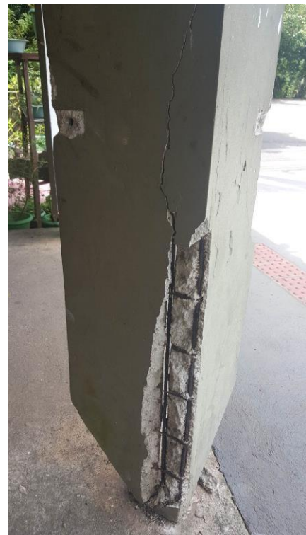
Fig. 8: Corrosion Process (Source: Author's Collection, 2019)
