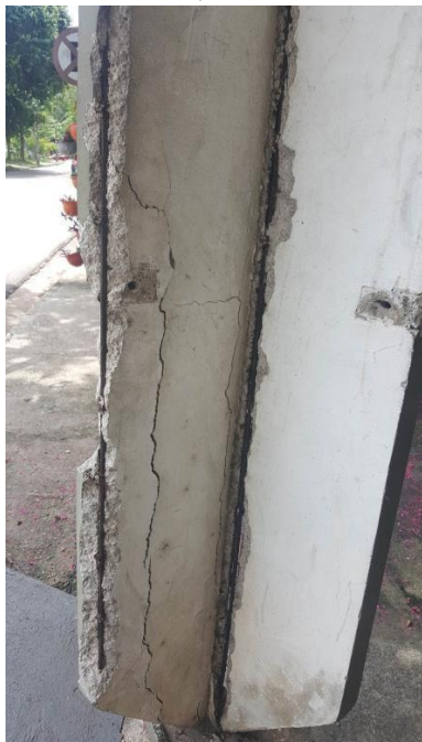
Fig. 7: Corrosion Process (Source: Author's Collection, 2019)
