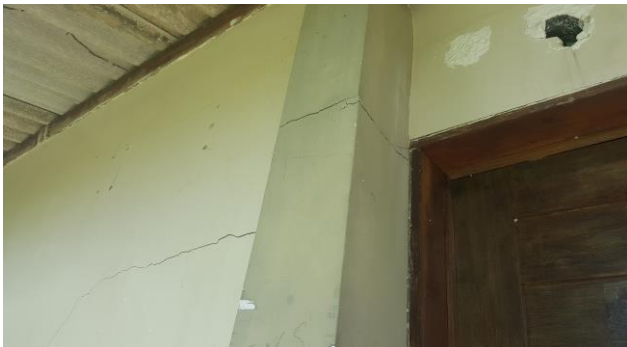
Fig. 10: Foundation Problems (Source: Author's Collection, 2019)
