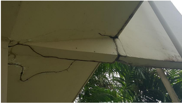
Fig. 5: Concrete segregation (Source: Author's Collection, 2019)
