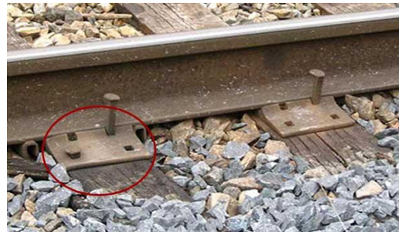
Fig. 1 Representation of (a) centered rail parts: tie plate (in cyan), tie (in yellow), and stay (in green). The round things on the tie plate are spikes, which affix it to the ground.
