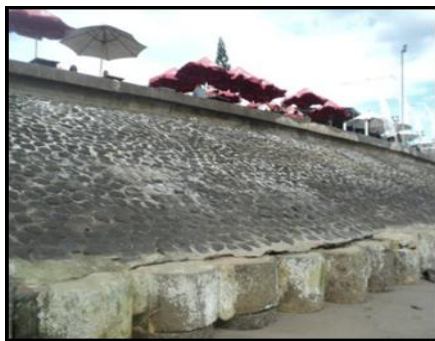
Figure 2. Seawall Crumbling Canggubali Beach, Bali, Indonesia (Nalarsih, 2016)
