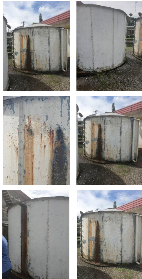
Fig. 1. Corroded storage tank surface
