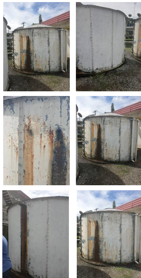
Fig. 1. Corroded storage tank surface
