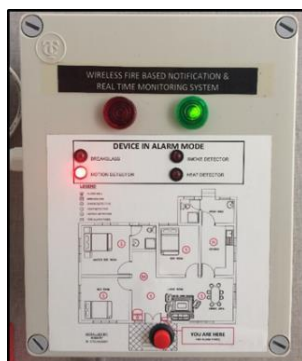
Figure 7. Normal Condition on Panel
