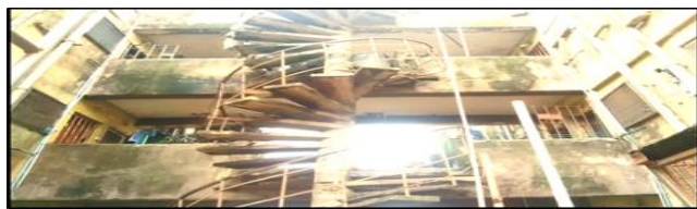
Figure 1: Balcony and staircase shared by occupants at Abesan Estate Source: Authors' Fieldwork (2016)
