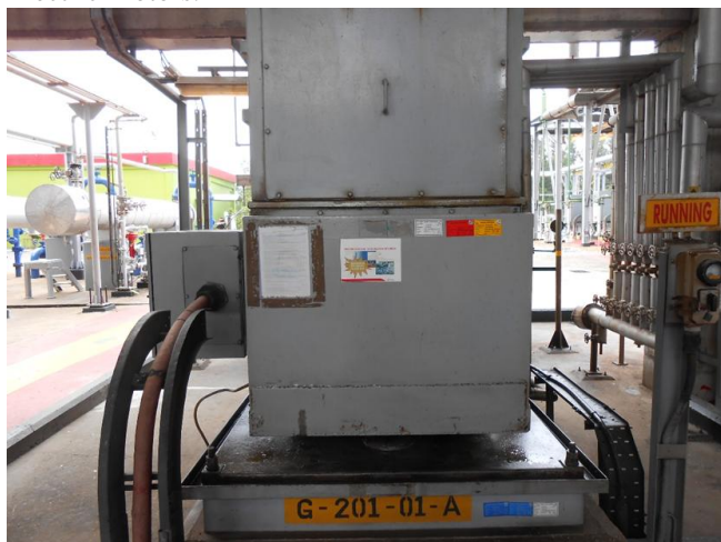
Figure 4. Control Systems on GM-201-01A Electric Motors
