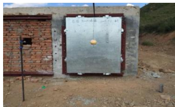
Fig. 10. Field Blast test set up of composite blast-resistant wall, Liang et al (2017)
