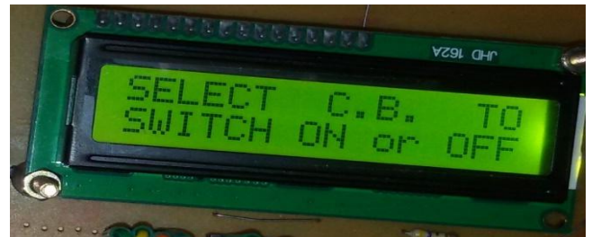
FIG. 5: IF THE CORRECT CARD IS GIVEN THAN IT WILL SHOW THE SELECT THE CIRCUIT BREAKER TO BE OFF
