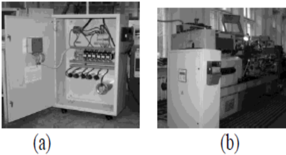
Fig.3. Automatic Reactive Power Control and Compensation devices ARPCC: (a). general view of ARPCC; (b). ARPCC connected to lathe 16K20
