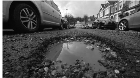
Fig. 10. Road damage due to natural calamities and vehicle movement
