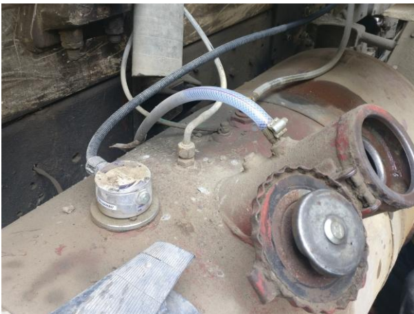
Fig. 6. Diesel fuel tank.
