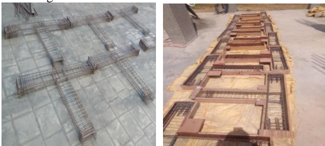
(a) Reinforcement details (b) Form work for casting Fig. 3: Reinforcement and Setup for casting
