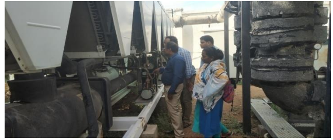
Fig.3.Field Visit Exposure on Centralized Air conditioning system
