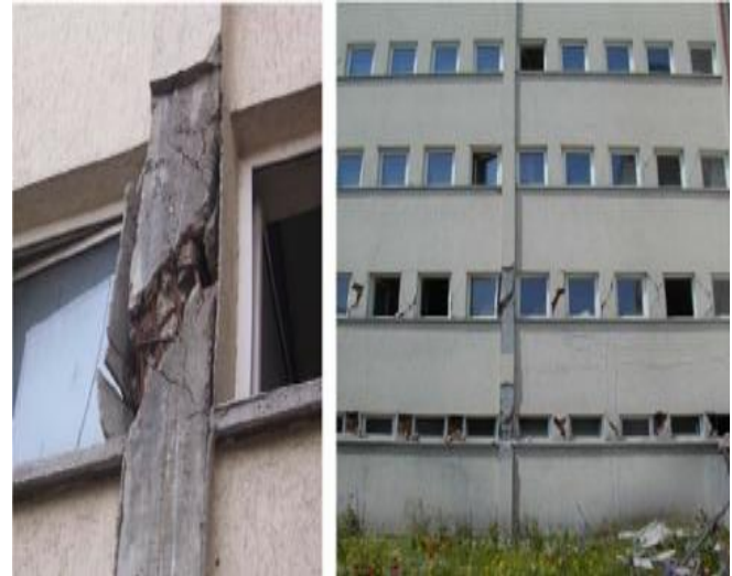
Fig. 1. Captive Column Failure
