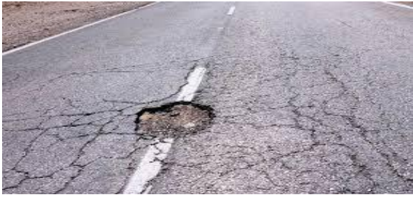
Fig 4 Cracks on the roads
