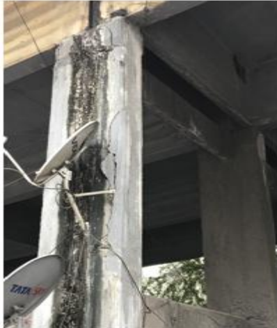
Figure 1:- Cracks in column number 6A due to satellite dishes.
