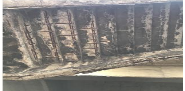
Figure 2. Exposed reinforcement on the underside of the staircase.
