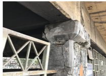
Figure 3. Structural cracks were seen on the columns
