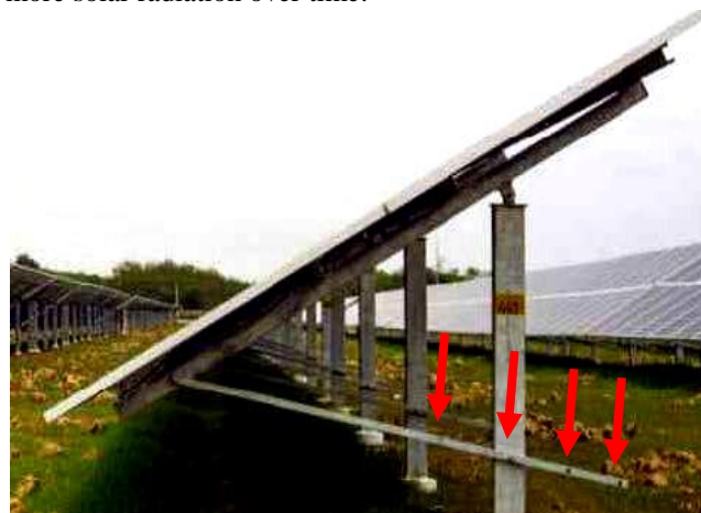
Fig. 4. Seasonal Tilt Solar Plant
