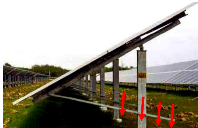
Fig. 4. Seasonal Tilt Solar Plant
